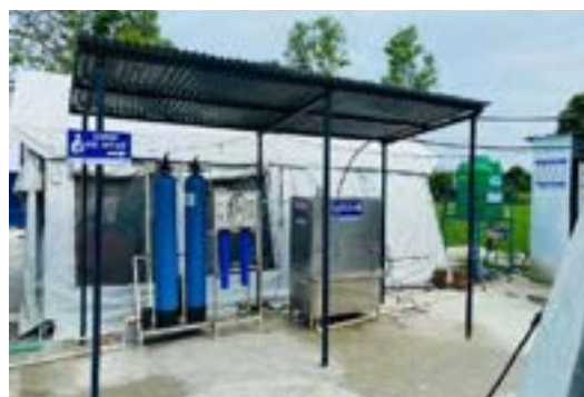
Clean and Safe Drinking Water facility at Health Desk- Gaddachauki
